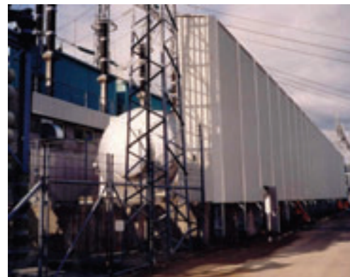
Substation acoustic screen
