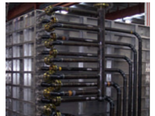
Dairy heat exchanger
