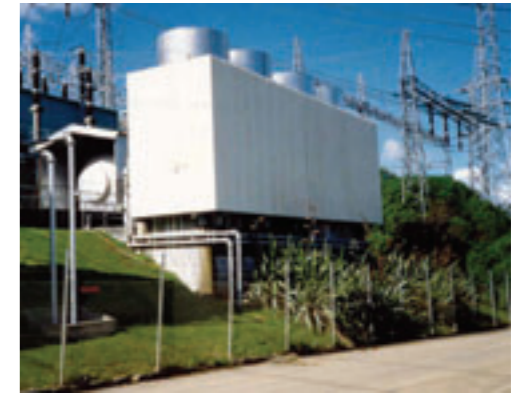
Cooling tower attenuators
