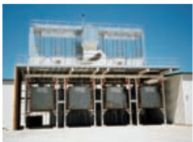
Modular filters at FCF Taupo mouldings plant.
